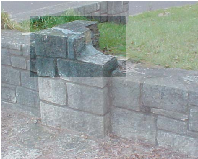
Missing stone(s) at wall pier
