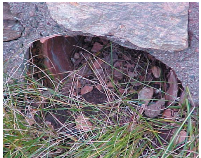
Original clay tile weep at base of wall
